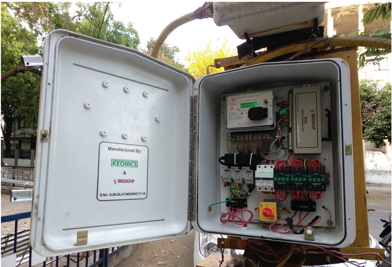
Figure 3: Central Control Monitoring System
